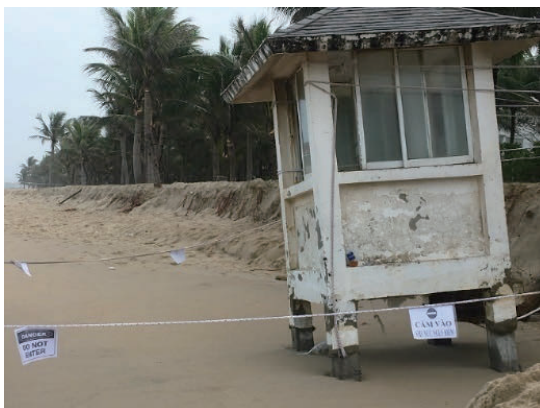
Figure 3. A corner of the guard house and fence of a resort were destroyed by waves (January 28 th , 2018)
